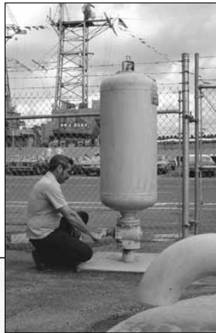
Refineries — Shock from pump starting and stopping
