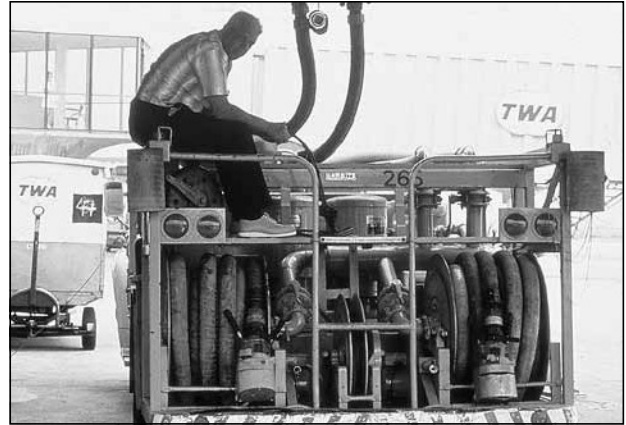
Protecting sensitive meters and small diameter piping from valve closure on fueling trucks
