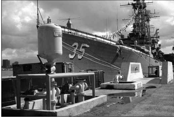
Fuel loading absorbs shock from pump startup and stopping
